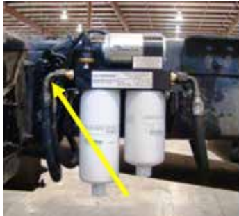
A curved 90° fuel line fitting was used with this installation.
