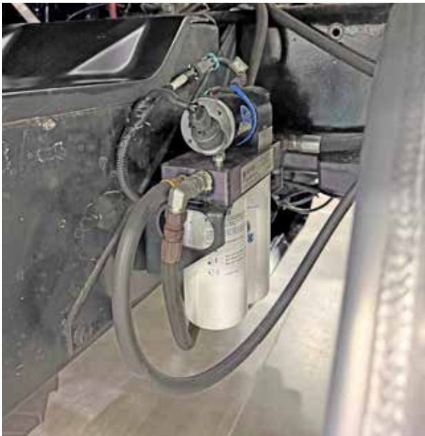
This installation on a short nose "Day Cab" is on the driver's side, behind the battery box.
