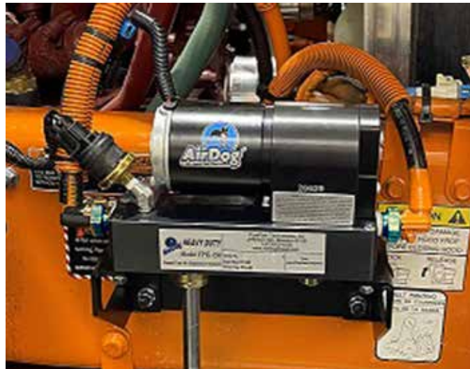
This example shows the AirDog® installed.
