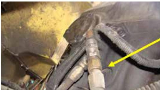
Engine Fuel Return Line
