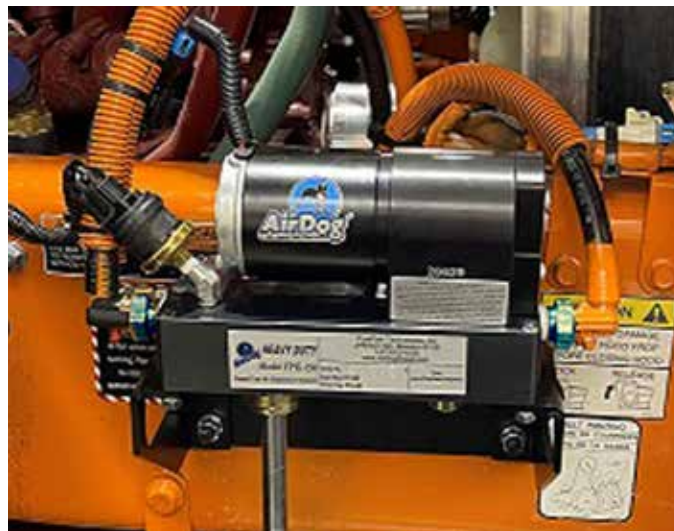
This example shows the AirDog® installed.
